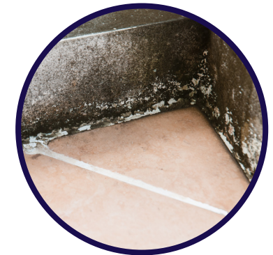
moulds and spores (damp, poorly ventilated housing)
